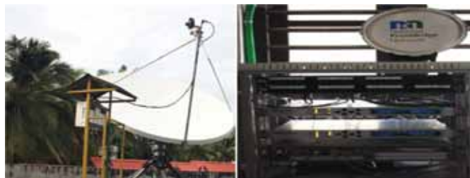
Figure: High Capacity SCPC VSAT at Kavaratti, the U.T. of Lakshadweep Island for NKN
