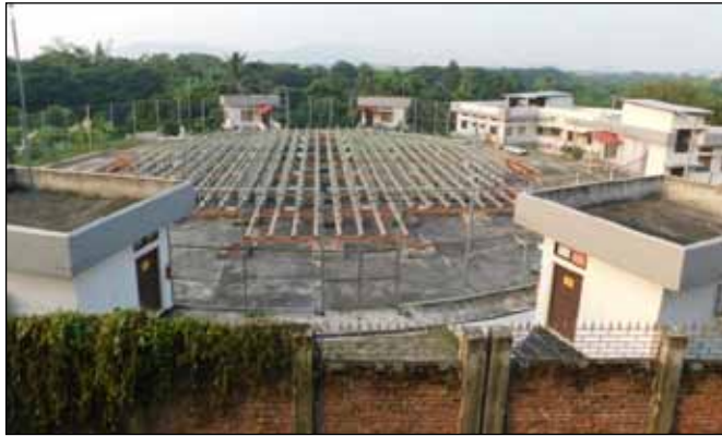
ST Radar site
